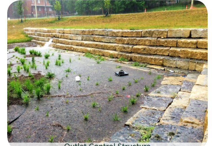
Outlet Control Structure
