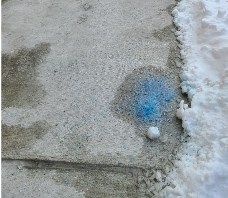
Figure 22. Region of high salt application which can result in surface scaling
