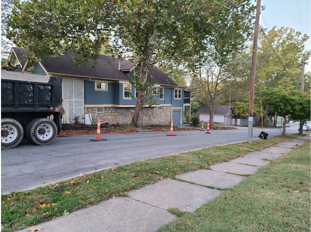
Figure 6. New sidewalk surface test section located along 41 st St. (Image looking to the southwest)
