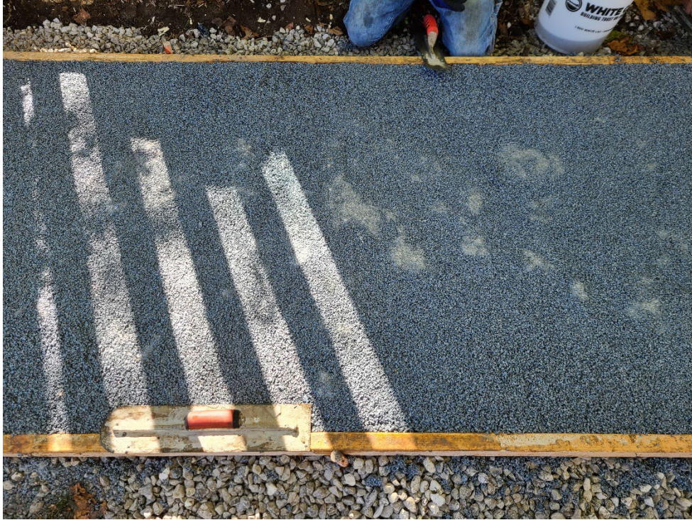
Figure 14. Bubbling of Rubberway as polyurethane reacts with ground moisture
