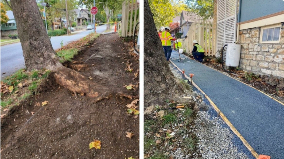
Figure 8. Tree root protected (left) before aggregate base installation, (right) after Rubberway placement
