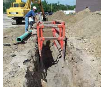
Sanitary sewer improvements in neighborhoods with clusters of septic systems will require creative approaches to limit the financial impact upon property owners.
