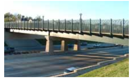
Future improvements to freeway interchanges should provide safe crossings and bridge railings suitable for both pedestrians and bicyclists, such as this example from Bruce R. Watkins highway (U.S. 71 Hwy) in Kansas City.
