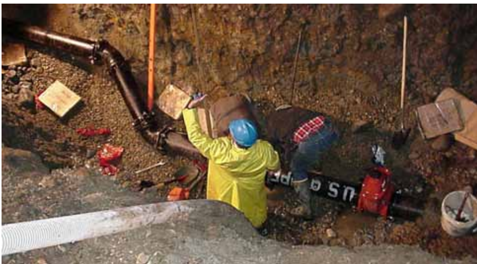
Water line improvements are needed in various locations in the Plan Area with undersized lines.
