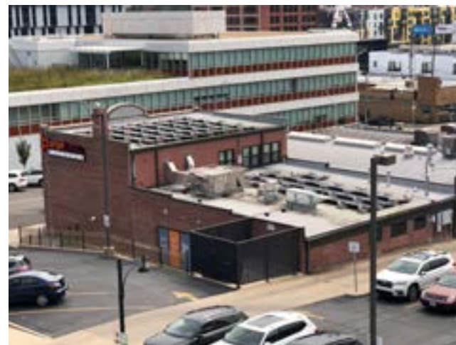
Solar Panels on Commercial Building 15
