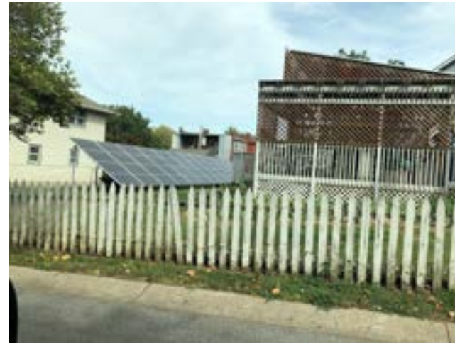
Solar Panel Array Freestanding 14
