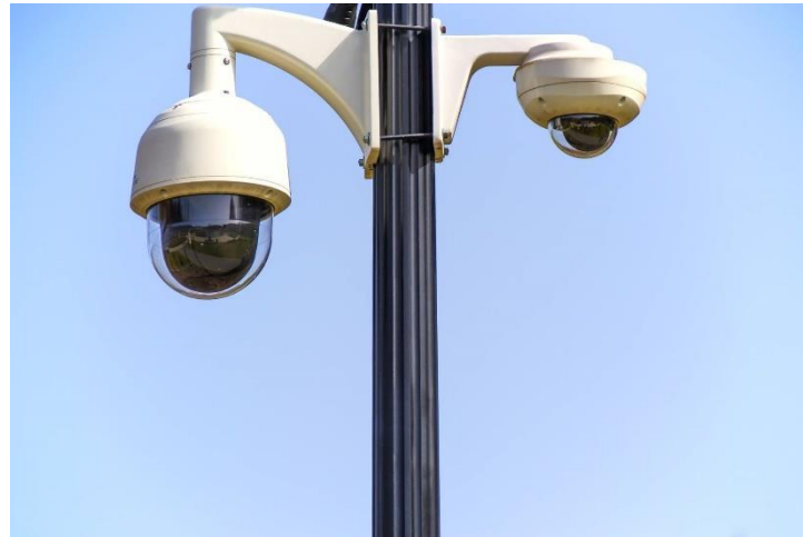
Cameras along corridor
