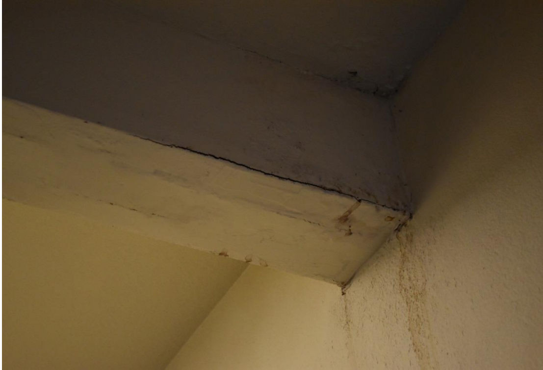
STAIR WELL – WATER DAMAGE FROM ROOF LEAKS
