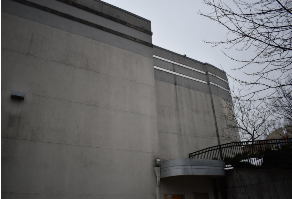
TWIN ELMS NORTH ELEVATION – NOTE STAINING FROM ROOF OVERFLOW.
