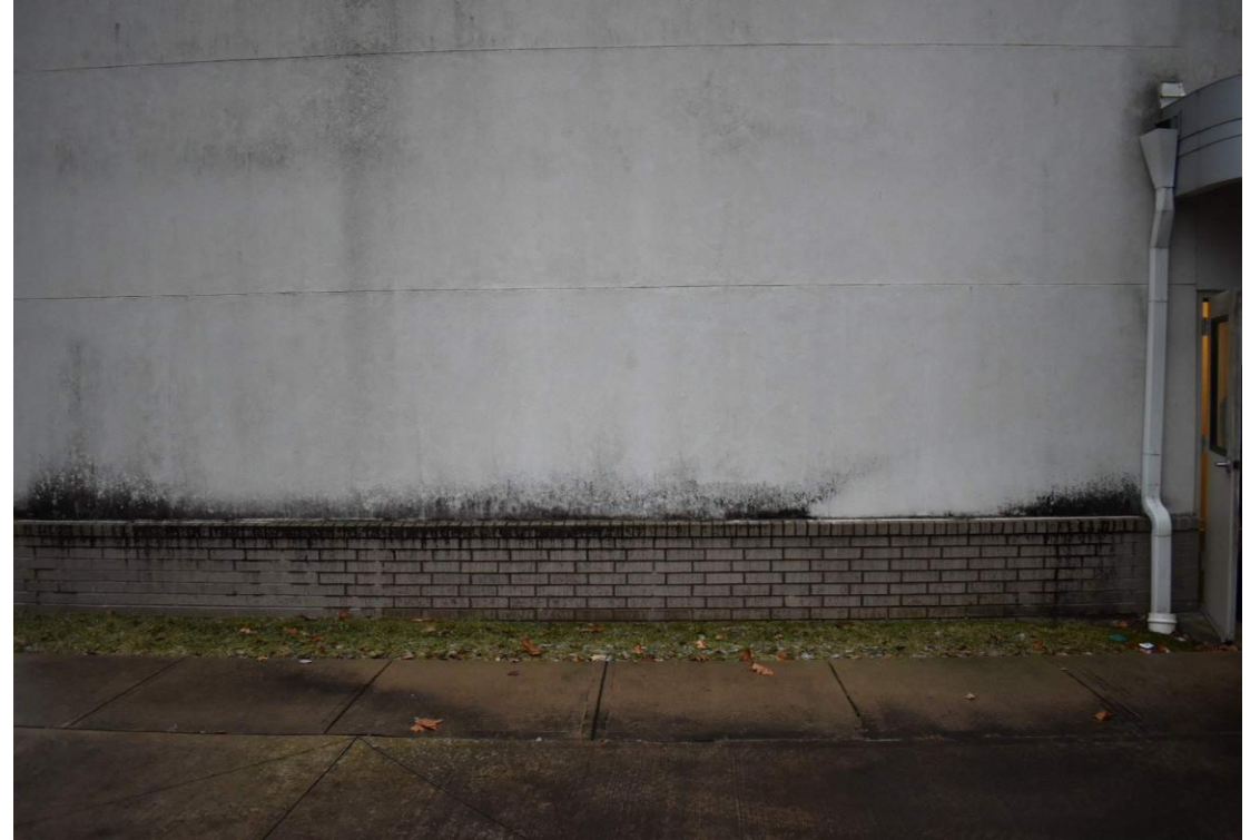
TWIN ELMS NORTH ELEVATION – STAINING ON WALL (TYPICAL) REQUIRING POWER WASHING AND REPAINTING.
