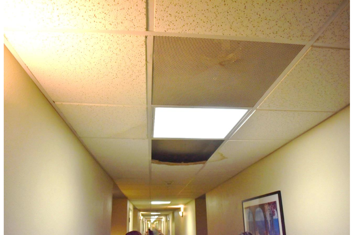
WATER DAMAGED TILES, 3 RD FLOOR CORRIDOR, DUE TO RECENT RAIN LEAKS. THESE AREAS HAVE BEEN PATCHED MULTIPLE TIMES.
