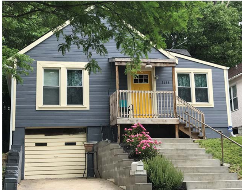
Photo of a rehabilitated home that received new siding and paint in a targeted neighborhood.
