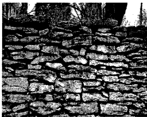
The joints in the photo on the left are quite noticeable, and should be preserved. A dry stack wall, however, should not have mortar added later.
