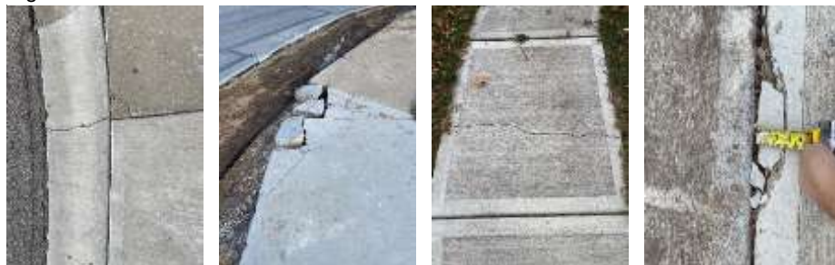
Figure 1. New Sidewalks with Defects
