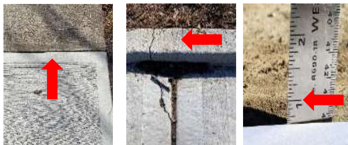
Figure 2. Joints with no old to new expansion, missing, or depth too shallow
