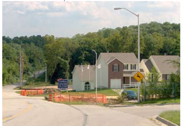
New construction continues to emerge on the edges of the previously undeveloped terrain.
