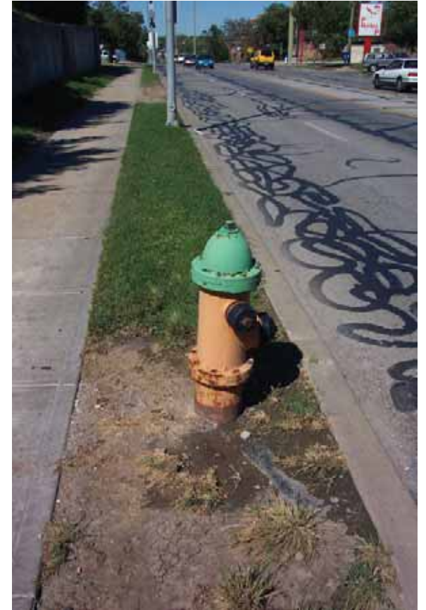
Fire hydrant in buffer area.
