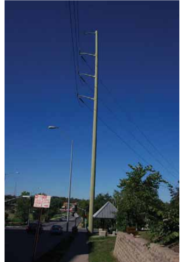
Major overhead electrical transmission lines.
