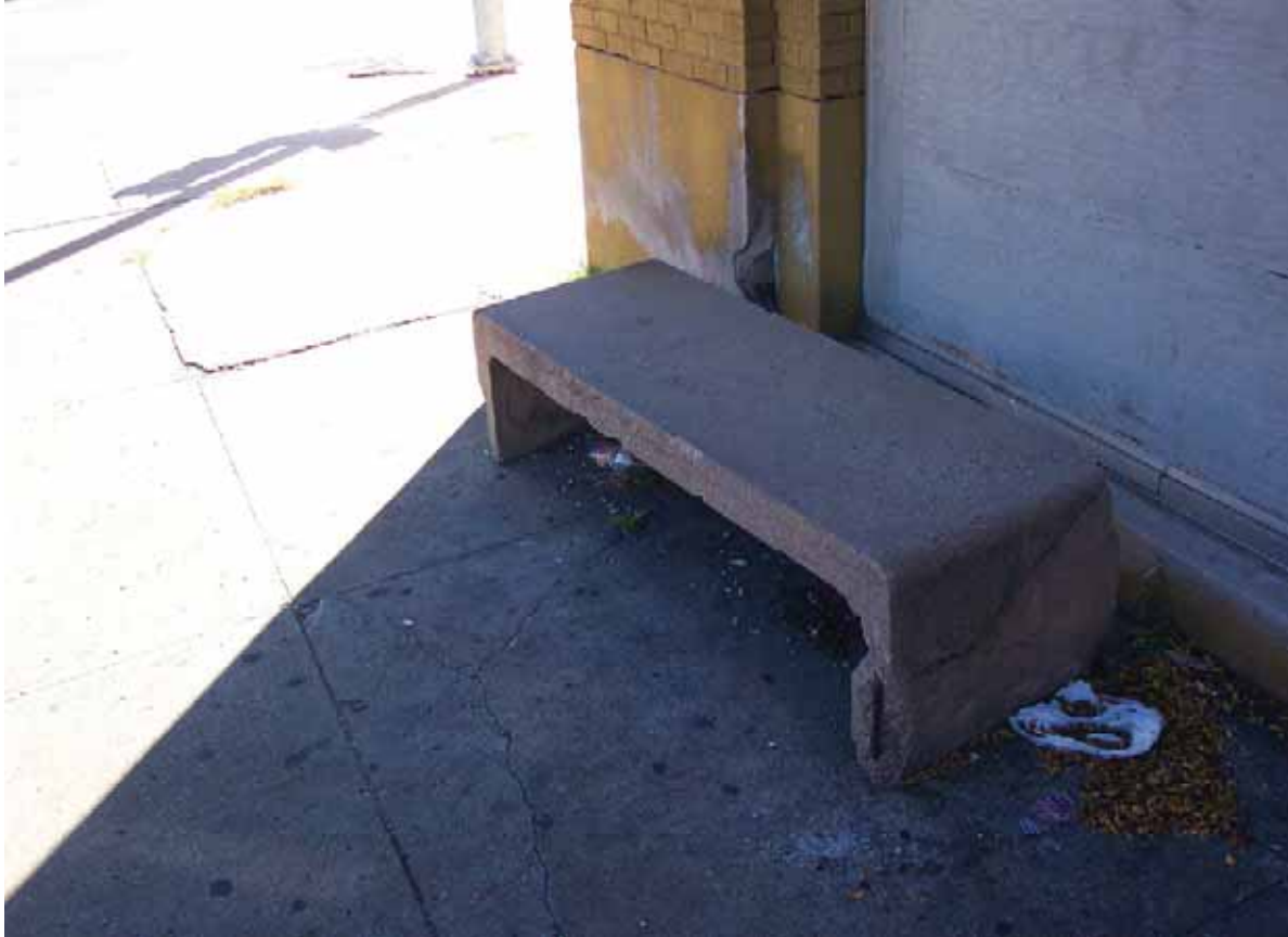
Site furnishings are inconsistent. Existing concrete bench is deteriorating. No trash receptacle is located by the bench and trash is evident. Broken glass remains at the trash receptacle.
