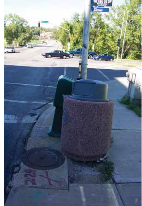
Vending machines and concrete trash receptacle with lid. Walk and drainage inlet are deteriorating.
