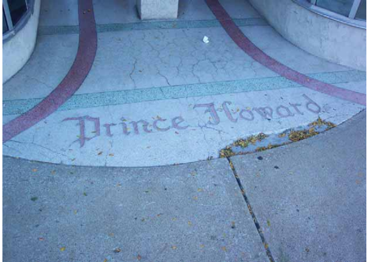
Special paving at Prince Howard entrance. Pavement condition is deteriorating.
