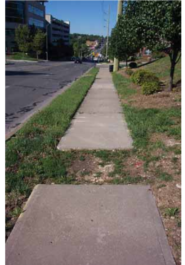
Gap in sidewalk.
