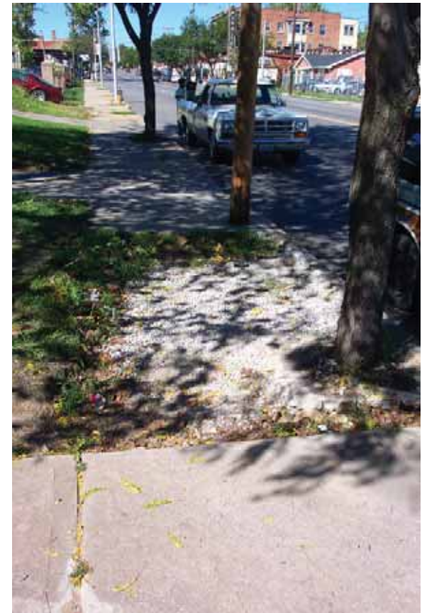
Concrete walk is not continuous.
