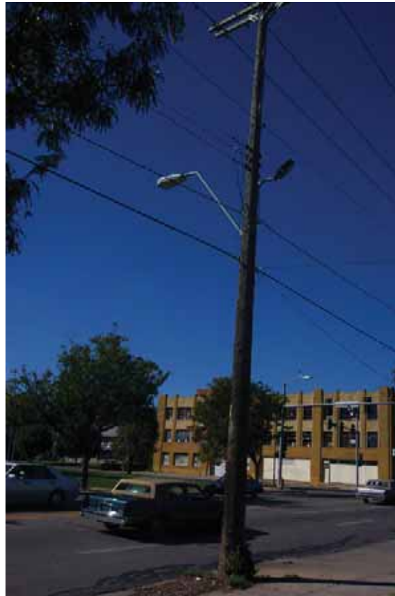
Wood utility pole and overhead utilities.
