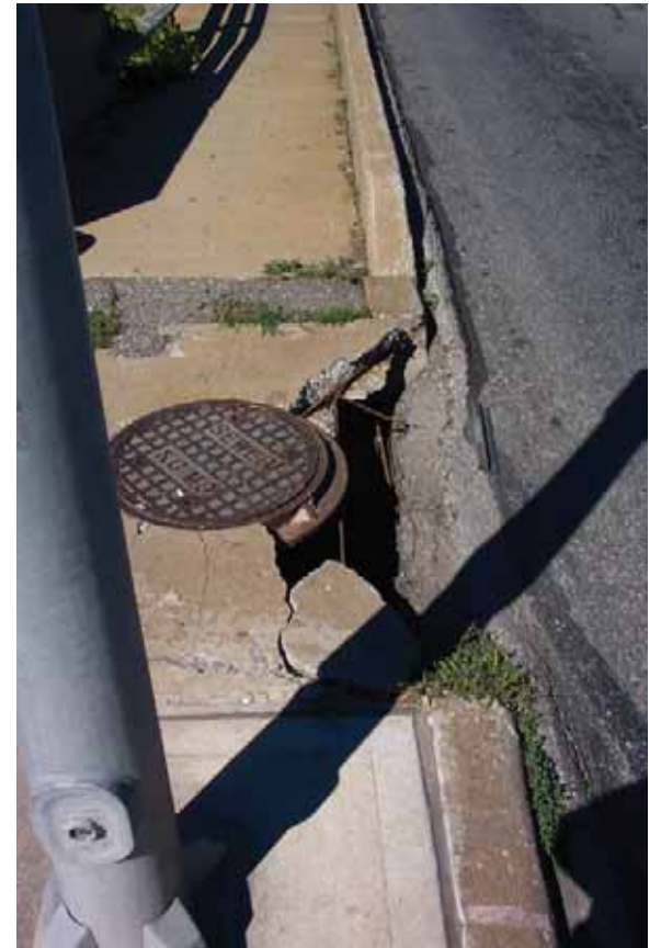
Damaged storm sewer inlet creating a safety hazard.
