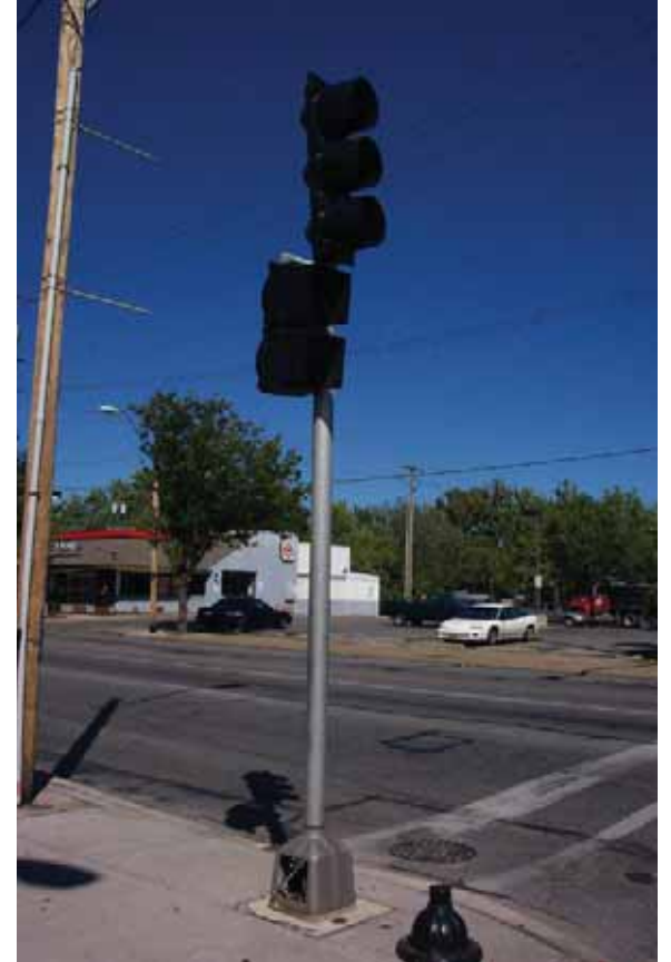
Traffic signal with pedestrian signal but missing actuator buttons.
