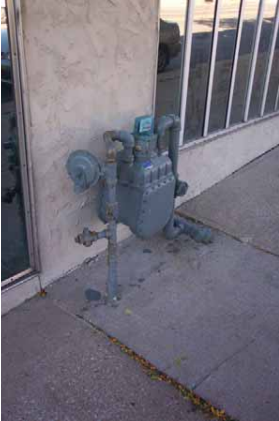
Gas meter visible from street.
