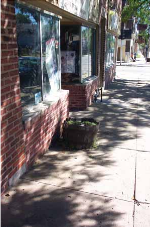
Storefront entrance with planter. Plantings are not maintained and planter is not consistent with materials on the storefront.
