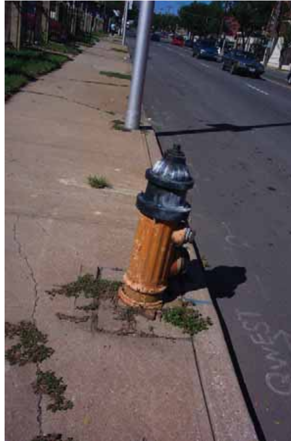
Typical fire hydrant and metal utility poles adjacent to roadway. Street trees are absent from one side of the corridor. Sidewalk pavement is deteriorating.
